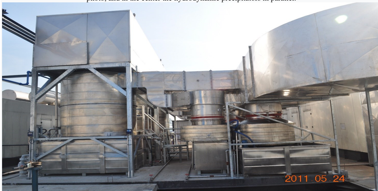
Figure 6- 12.5 MW cogeneration plant, expansion plenum, and primary combustion gas quencher on the left of the photo, and in the center the hydrodynamic precipitators in parallel.
